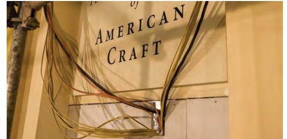
Well, we knew the electrical system needed to be upgraded.
